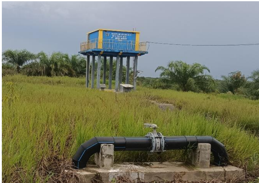
Clean Water Storage Facility Managed by the Community
