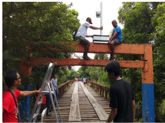
(b) Installation of the solar lighting system on both sides of the bridges
