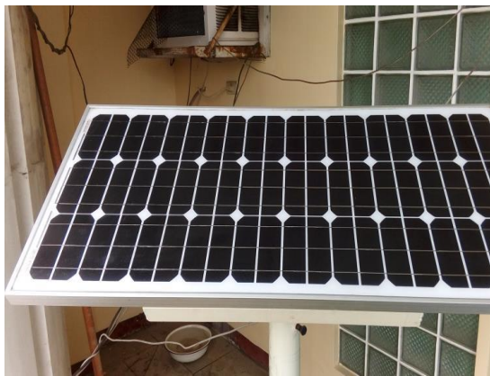
(a) Solar panel unit (80 W / 26 A) capable of charging the battery even in mildly sunny conditions
